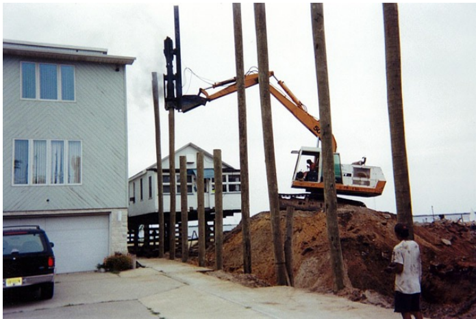
Highlands, NJ Pile driving a New Jersey shore dwelling utilizing a diesel hammer. This method allows us to get piles driven in tight work spaces.
