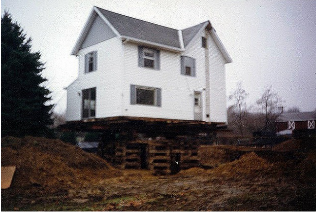
Brielle, NJ A shore home located in Brielle, NJ that had to be moved to the bay while contaminated soil was removed and a new foundation constructed.
