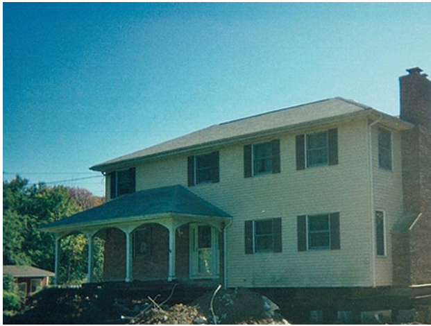
New Jersey This dwelling was elevated in place to create a tall, full basement and to alleviate flood problems.
