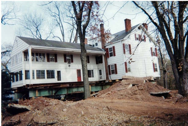
New Jersey This house with five chimneys was moved approximately 750 feet up a hill to escape from a flood zone area.
