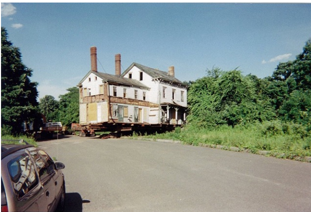
Orange, NJ This structure was moved to allow for a contaminated oil container to be removed from the ground.
