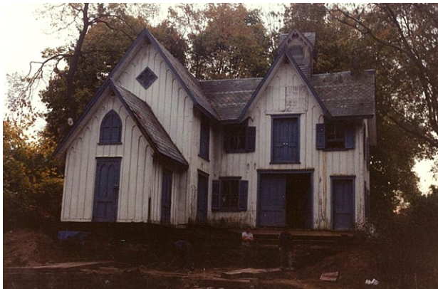
Upstate, NY This historic structure in upstate New York that was raised to repair the sills and foundation.
